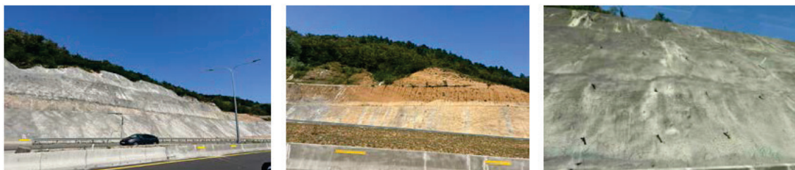
Fig. 3. Some examples of cut slopes caused by road widening at the Rikoti crossing.
